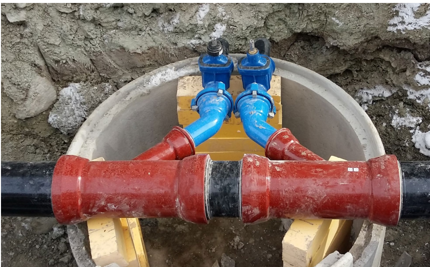
ECOPUR DN 250 with house infeed DN 100 to the heat exchanger
